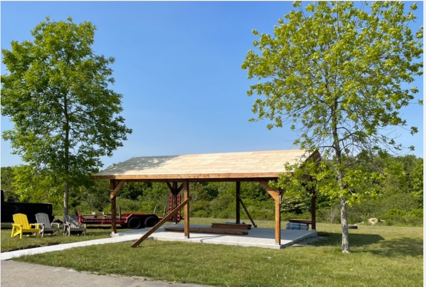
Pictured above: a new outdoor learning space was recently constructed at Drumlin Heights Consolidated School.
